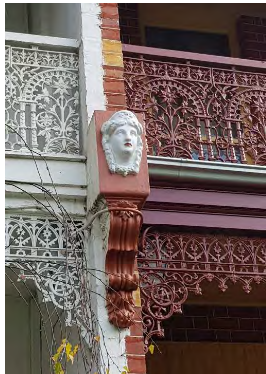
Figure 472. The moulded detail with sculpture relief on a party wall. (Source: GML Heritage, 2022)
