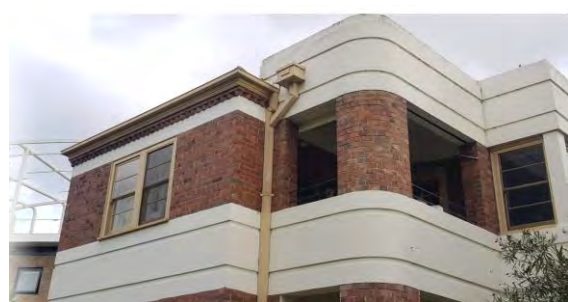
Figure 359. Detail of the upper storey of the southern wing showing the face brick, render, and curved balconies. (Source: GML Heritage, 2022)
