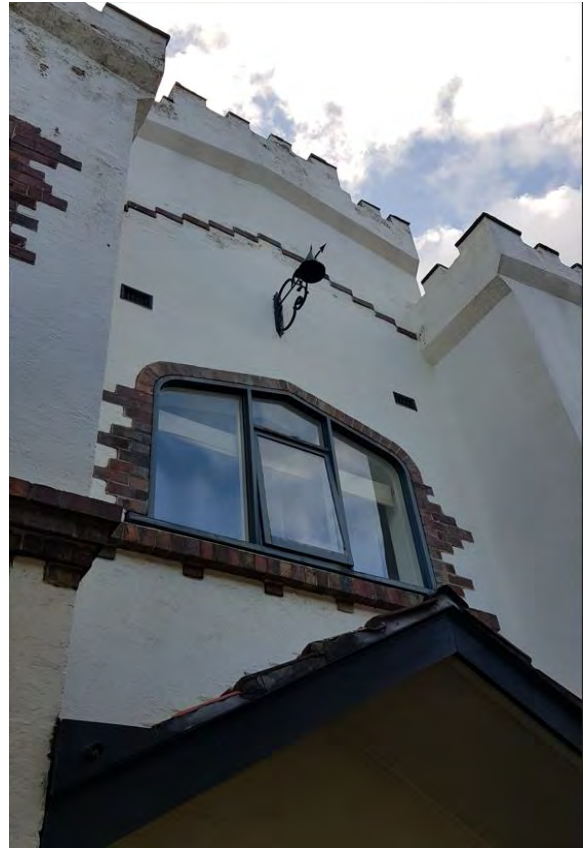
Figure 423. Detail showing a Tudor arched window, and the crenulated battlement style parapets. (Source: GML Heritage, 2022)
