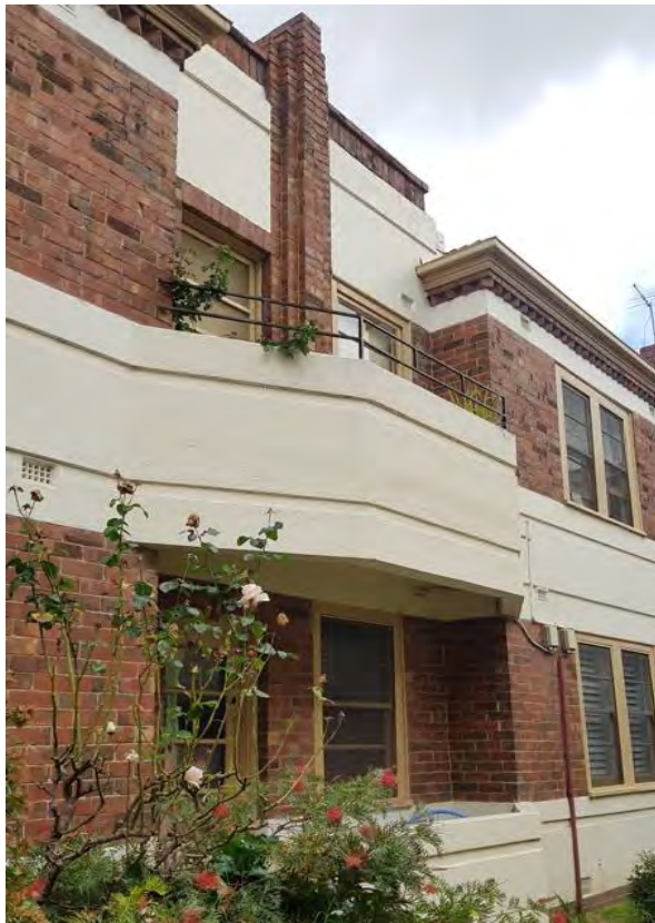
Figure 360. Detail showing a faceted balcony in the central courtyard. (Source: GML Heritage, 2022)
