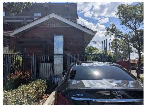
Figure 165. Northern substation. (Source: GML, 2023)
