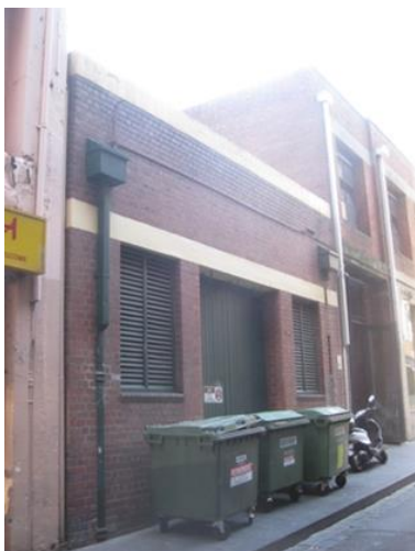
Figure 5. Substation at 28 Crossley Street, unknown build date.
