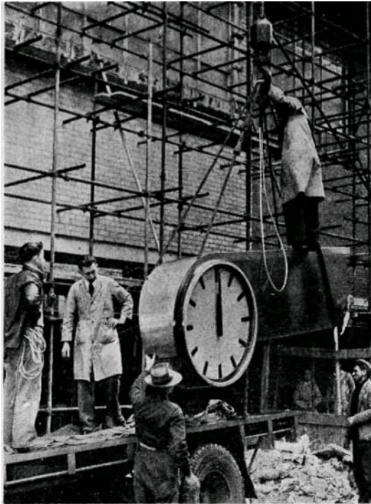
Figure 4. Extract from photograph showing the 6cwt (approximately 300kg) timepiece being installed at Russell Street Exchange building in 1954. (Source: Age 23 July 1954:8)
