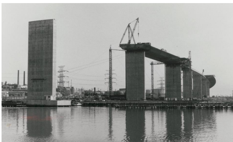
Figure 4: The West Gate Bridge under construction, photographed by John T Collins on 20 September 1970, less than a month before the tragic collapse of a span (SLV H98.250/2167, http://handle.slv.vic.gov.au/10381/234189 )
