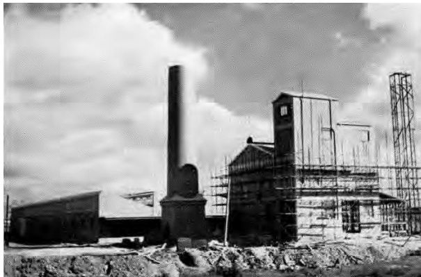
Figure 5: Captioned 'a Victorian dehydration factory' this is the Fishermans Bend boiler house under construction in 1943, with the sawtooth roof of the dehydration factory building behind (Allied Works Council, 1943, p.73)
