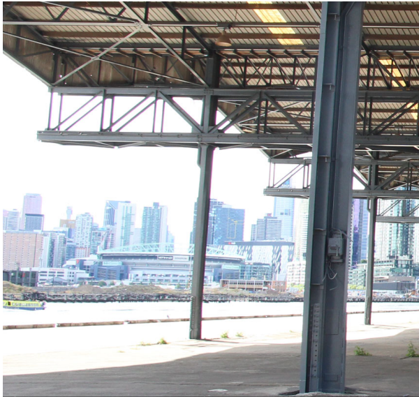
Figure 7: The flat, parallel chord trusses originally extended past the building towards the Yarra River, and were supported on columns that have now been severed. They once supported the seven bridge cranes that have been removed. The reinforced extension of the columns can be seen near the base (P Mills, 03/04/2018)
